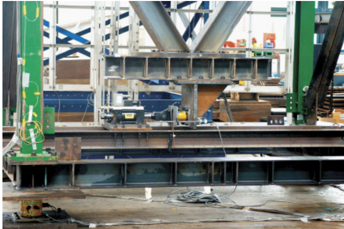
Figure 12. A RSASD installed in the first storey.
